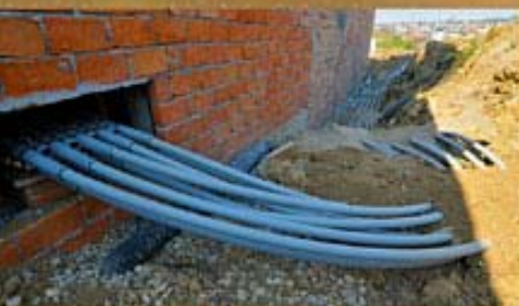
Connection of the vertical geothermal probes to the underground parking
