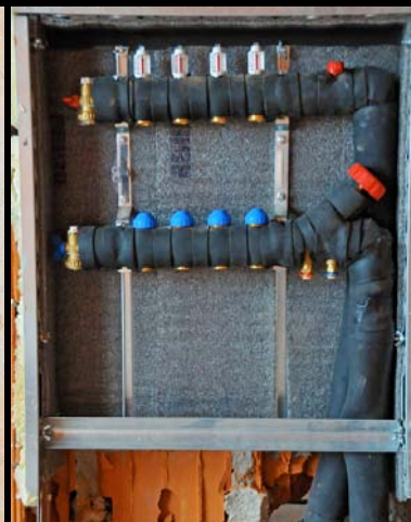
Insulation of pipes (thermal and noise protection)
