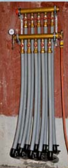
Grouping of the probes before connecting to the heat pump
