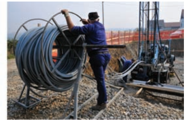
Početak spuštanja geotermalne sonde u bušotinu. Starting the descent of the geothermal probe into the borehole.
