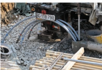
Sonda instalirana u bušotinu. Dužine je 100m i 1m ostaje vani za povezivanje. The probe installed in the borehole. It is 100m long and 1m stays out to connect it.
