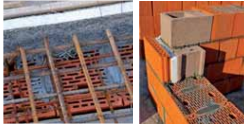
Figure XV.vi - Placing horizontal and vertical cerclage elements with thermal insulation on Apartment house Amadeo (photo Kuće Beodom, www.beodom.com )
