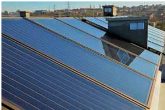
Figure XV.viii - Solar thermal panels on the roof of Amadeo building (photo Kuće Beodom)
